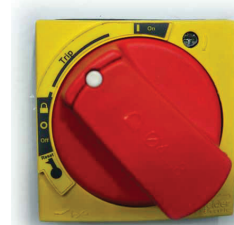
Fig. 60 Circuit breaker tripped
