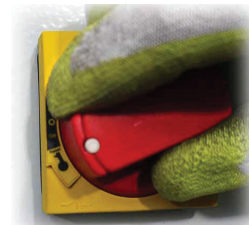
Fig. 61 Resetting the circuit breaker
